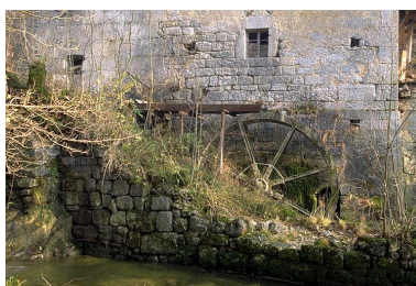
Roue hydraulique verticale aval. Phot. Laurent Poupard IVR43_19913901265ZA
