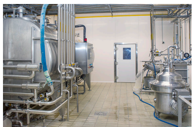
Salle de la station de lavage CIP. Phot. Sonia Dourlot IVR43_20142500759NUC2A
