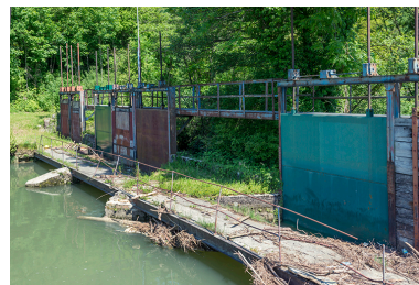
Vannage du canal. Phot. Mary Ruffinoni IVR43_20132500617NUC4A
