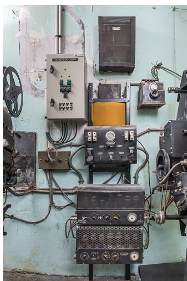
Installation de sonorisation. Phot. Pierre-Marie Barbe-Richaud IVR26_20222100057NUC4A
