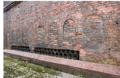
Orifices des tubes de la chaudière. Phot. Yves Sancey IVR43_20092500343NUC2A
