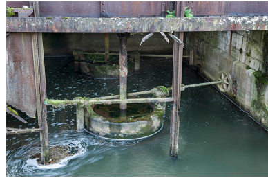
Turbines Douge. Phot. Jérôme Mongreville IVR43_20142501648NUC4A
