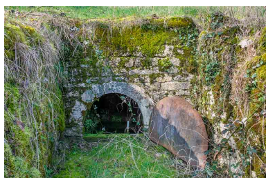
Captage de la source. Phot. Jérôme Mongreville IVR43_20243900533NUC4A
