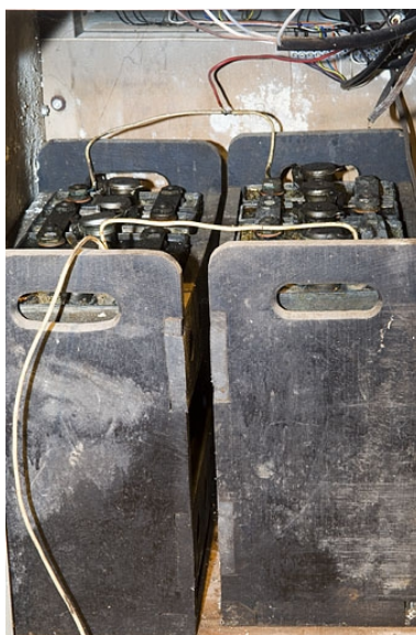
Les batteries. Phot. Jérôme Mongreville IVR43_20072501074NUCA
