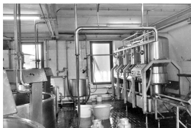
Installation de soutirage. Phot. Laurent Poupard IVR43_19913901175Z
