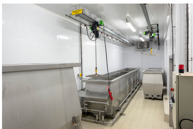
Bain de saumure. Phot. Sonia Dourlot IVR43_20182501705NUC4A
