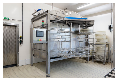
Installation de lavage. Phot. Sonia Dourlot IVR43_20192500956NUC4A
