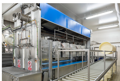
Installation de moulage. Phot. Sonia Dourlot IVR43_20192500919NUC4A
